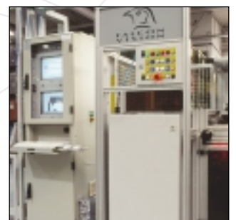
In-line measurement system
